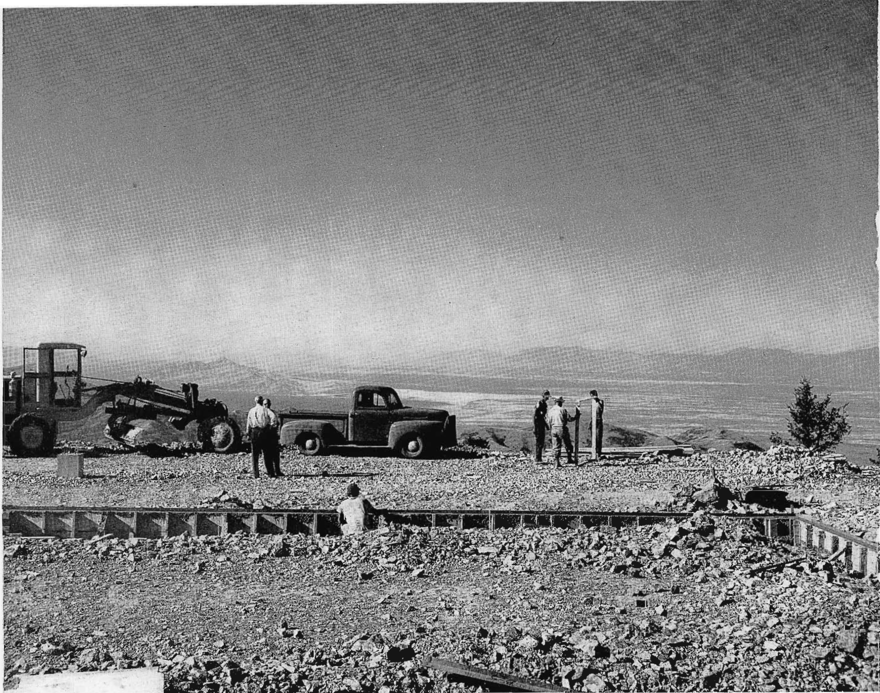
FIG. 3. Before construction could start it was necessary to bull-doze a flat place on the ridge. This is a view looking north from the building site. Southern Idaho is visible in the distance. KDYL-TV covers 87% of Utah, as well as parts of Idaho, Wyoming and Nevada.
