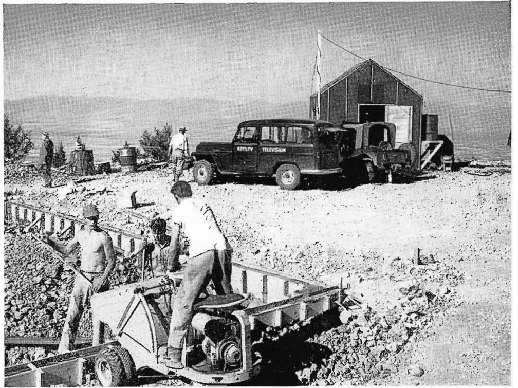
FIG. 4 (right). Another view of the mountain top taken during pouring of the foundations. All the construction materials and equipment were, of necessity, hauled over a temporary road having grades as high as 25% in places.
