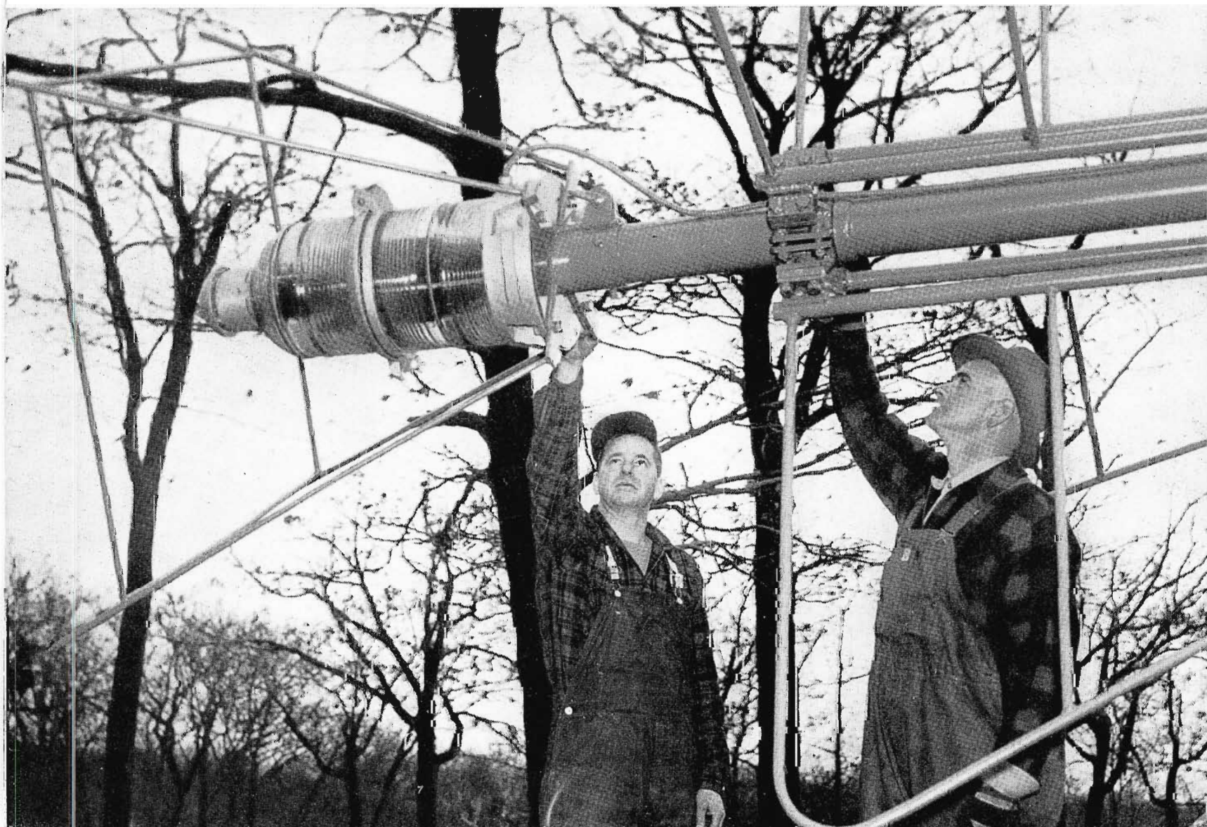
FIG. 5. A closeup view of the lightning protector arrangement which was built on the standard beacon mounting flange. Emile Racine of Racine Tower Construction, who assembled and erected the antennae, is shown at right with one of his men.
